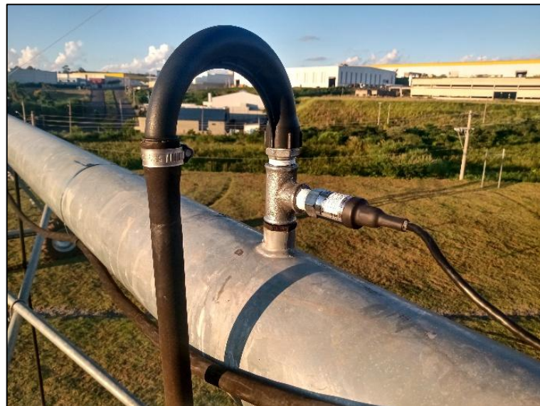
Figure 14 - Mechanical Installation of the Pressure Sensor.
