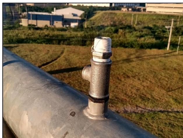
Figure 18 - Connection of the reducing tee and pressure sensor nipple to the pivot pipe.
