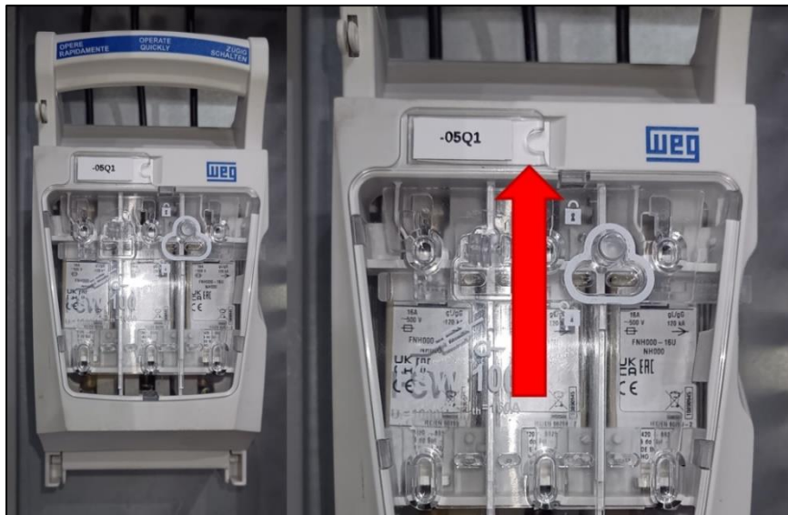
Figure 19 - Fuse puller switch in the locked position.
