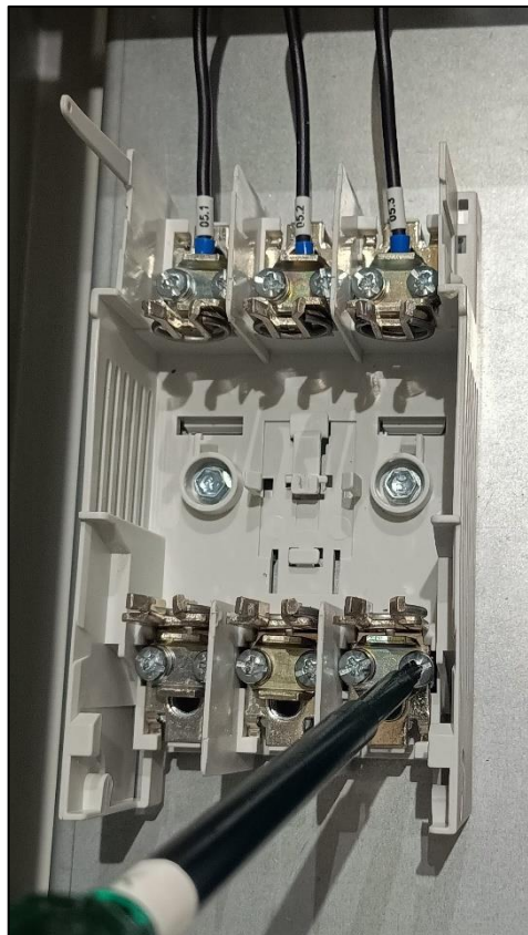
Figure 7 - Screws of the cable fastener.
